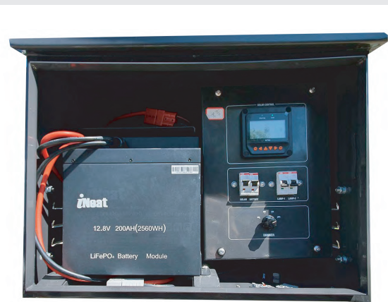
Battery and Control Box
