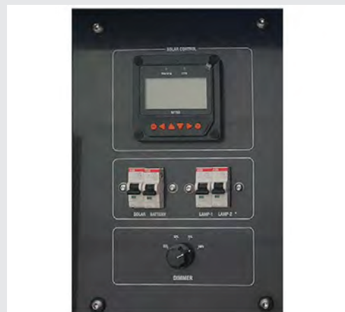
System Control Panel
