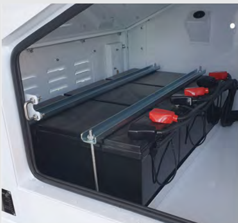
3 x 200ah LiFePO4 Batteries
