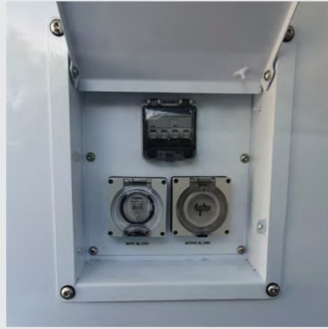
Inverter & 240V Charger
